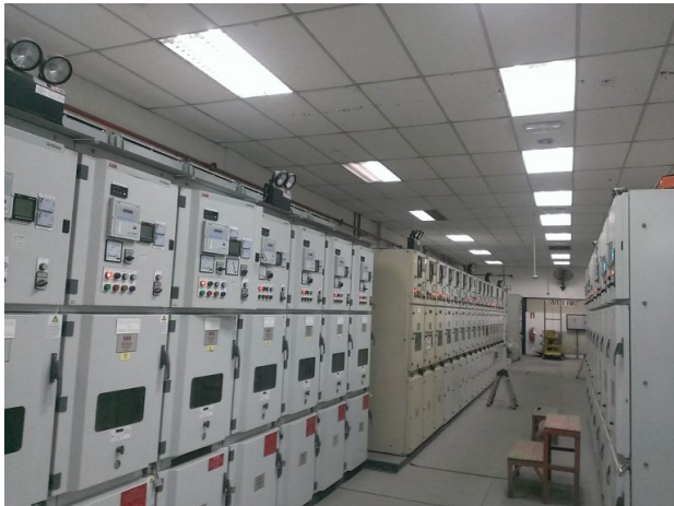
One of the many rows of power meter panels in MHB power facility room
