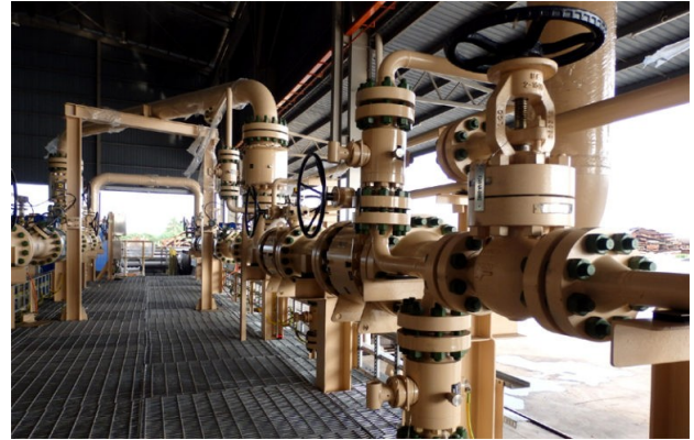
Fairview gas metering skid in post assembly stage
