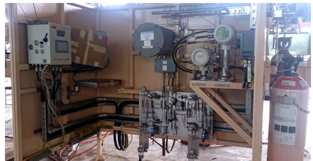
The analyzer shelter for Fairview gas metering system (which consists of Gas Chromatograph, Moisture Analyzer, Flow Computer, etc.)
