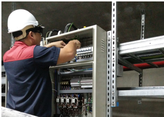
Technician troubleshooting a lighting DB panel in the bridge.
